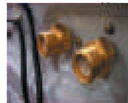
Brass Pressure Regulators installed on back of appliance.
